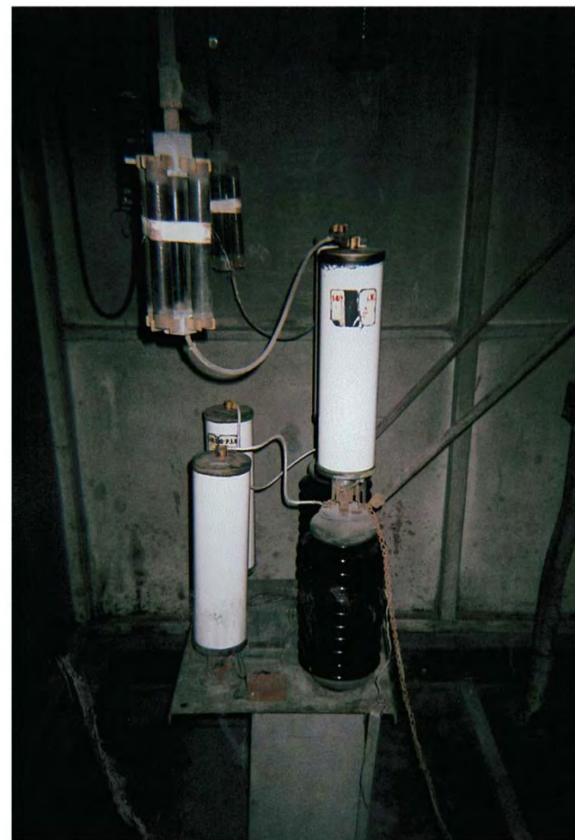
External Solid State Rectifiers Replaced Vacuum Tube diodes
